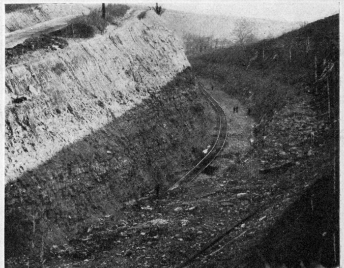
One of the Many Deep Cuts on the First 17½ Miles, Showing the Rock Penetrated
