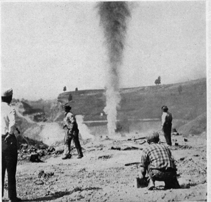
Some contractors sprung the holes used to blast cuts. Here's one in the section across the valley from McCabe's Cut looking towards Connellsville.
