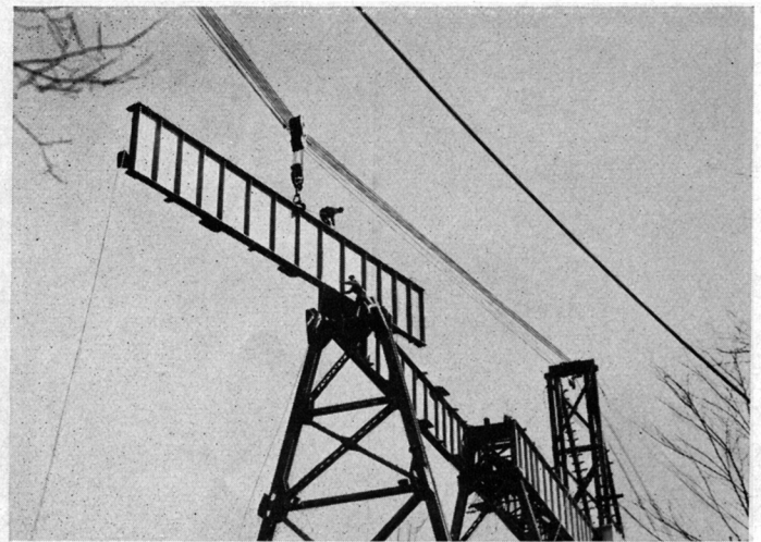
Probably the most spectacular part of this job was that of the steel men in erecting viaducts and bridges. A side plate on the viaduct over Maple Creek is sliding into place, directed by McClintic-Marshall bridge men.
