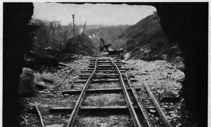
When photographed only the heading had been started in the short tunnel on the Donora spur. The view emphasizes the difficult terrain traversed.
