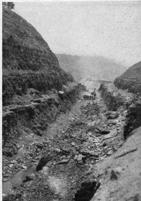
Near the junction of the Donora Southern connection is McCabe's Cut, one of the largest along the line. It was excavated by Jim McCabe, who used well drills and black blasting powder for drilling and blasting with great success.
