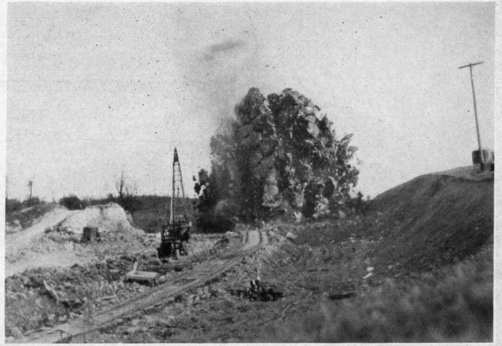
Near Finleyville, this blast in one of the cuts included 3,450 lb. of 40% dynamite. The charge was loaded in well-drill holes of 18 ft. to 20 ft. in depth.
