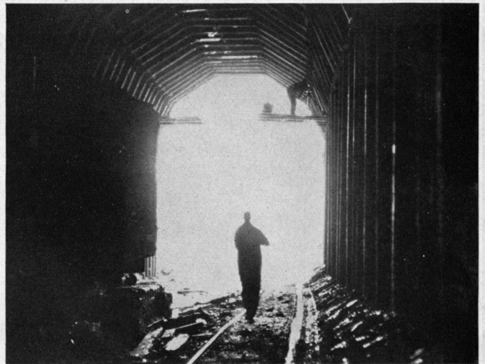
How timbers were set in the main line tunnels is revealed by this view out a portal. To the left is one of the shovels employed in mucking bench material.
