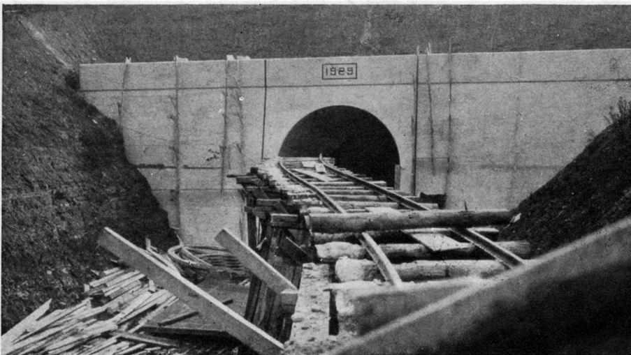
Portal at Pittsburgh End of Tunnel. An Especially Fine Concrete Finish Was Obtained Here
